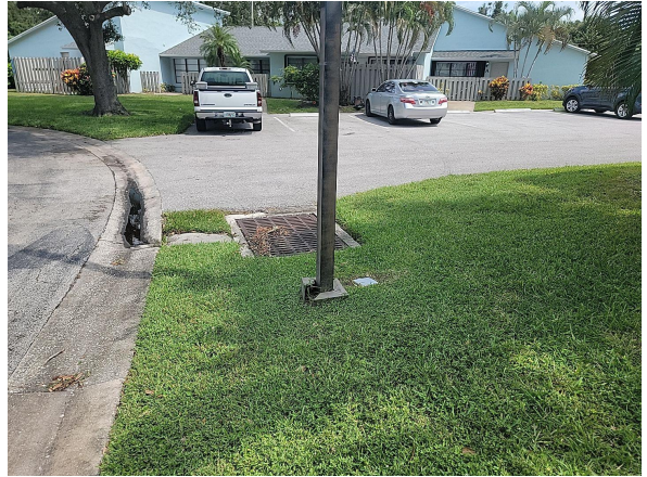
Damaged protective base
