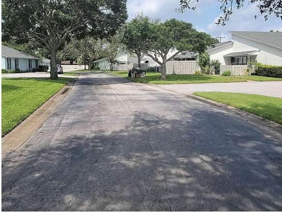
Worn asphalt paved street
