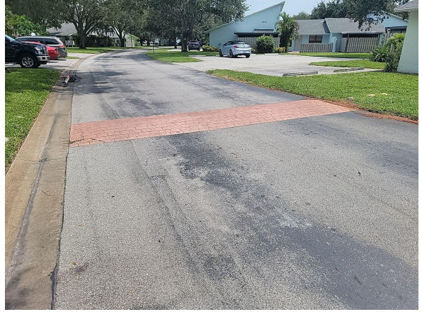
Damaged speed bump
