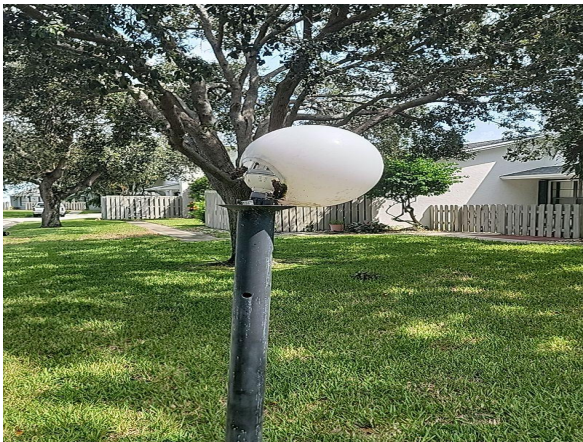
Damaged post lighting
