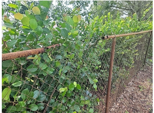
Damaged chain-link fencing
