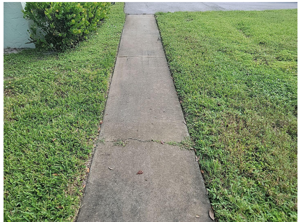
Damaged concrete walk
