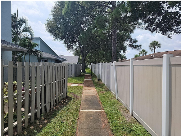
Damaged vinyl siding
