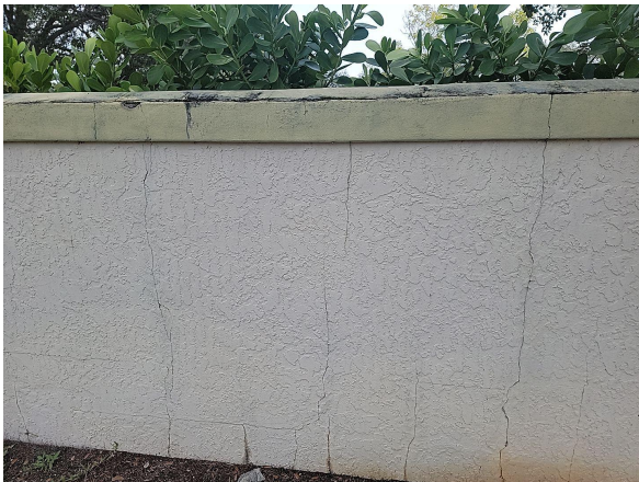
Damaged block and stucco perimeter wall
