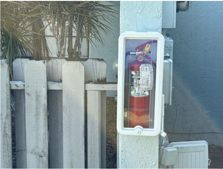
Photos / Fire Protections
